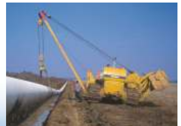
Paradip Haldia Pipeline
