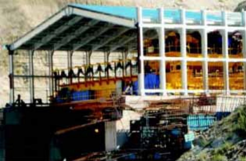
Kolar Dam Power House
