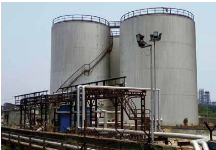
Heated bitumen tanks at Haldia Terminal
