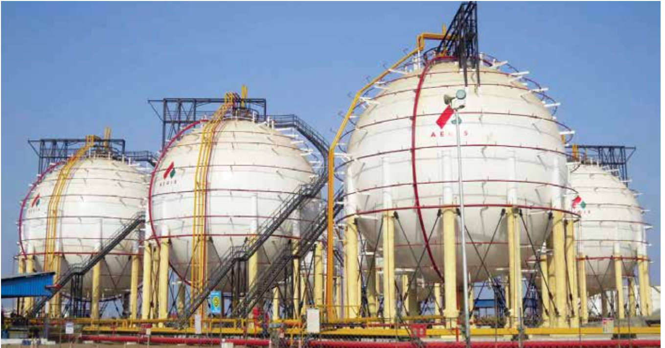
Newly commissioned LPG spheres at Pipavav
