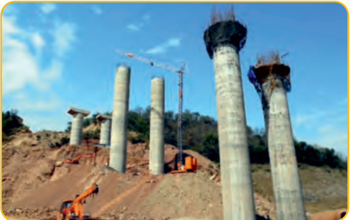
Sub structure work in progress at Km 26.184 Major Bridge at Kiratpur – Ner Chowk Road Project, Himachal Pradesh
