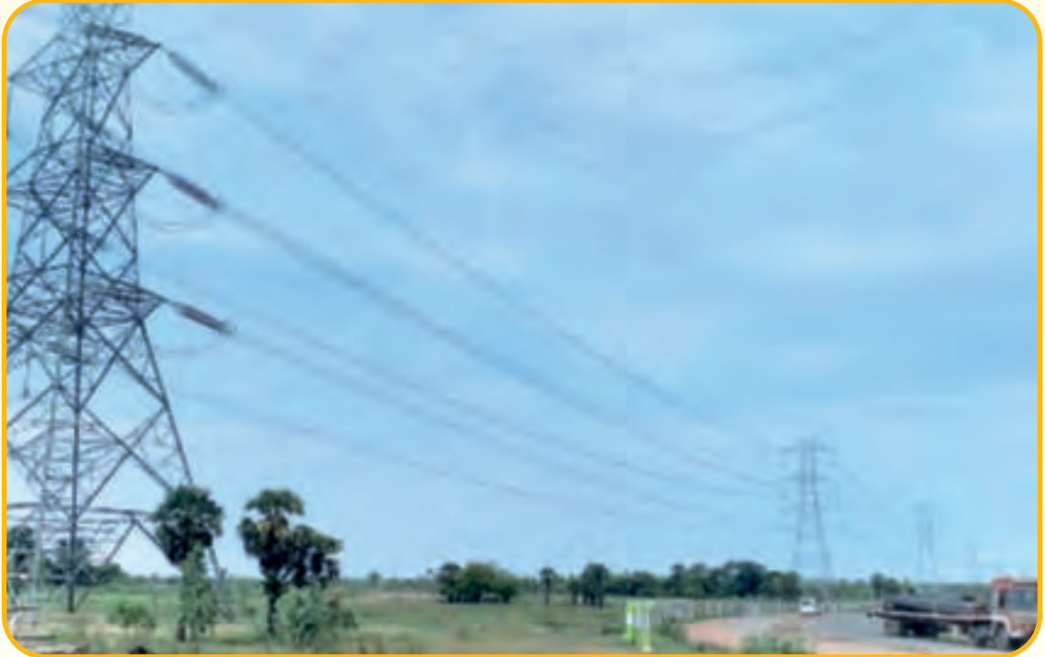
400 KV Double Circuit, Quad Moose Conductor and Suspension Tower at Cuddalore Transmission Line Project in Cuddalore District of Tamil Nadu
