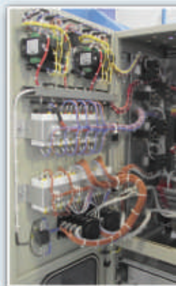
Power Distribution System
