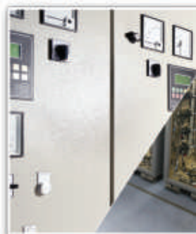
Marine Switch Board/Radar
