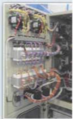
Power Distribution System
