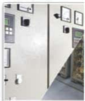
Marine Switch Board/Rack
