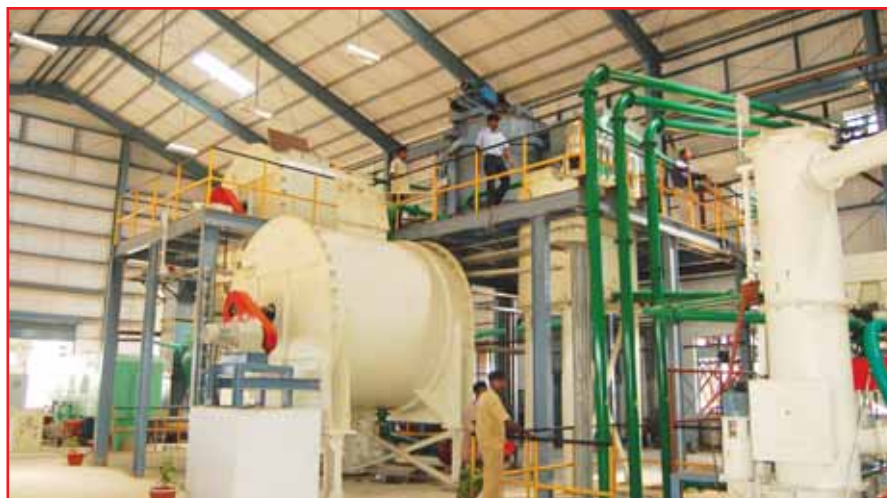
Slurry preparation Section at the Gangaikondan Plant
